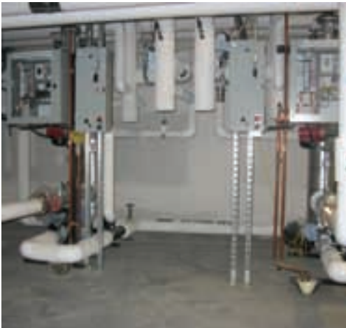
Domestic: 100 US gpm ; 40° F → 140 ° F Steam @ 125 psig ; Floor space 3' x 2' Back pressure 5 psig
