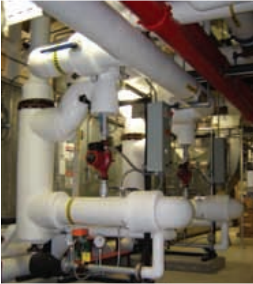
Building Heat: 440 US gpm ; 160° F → 180 ° F Steam @ 60 psig ; Floor space 4' x 2' Back pressure 8 psig
