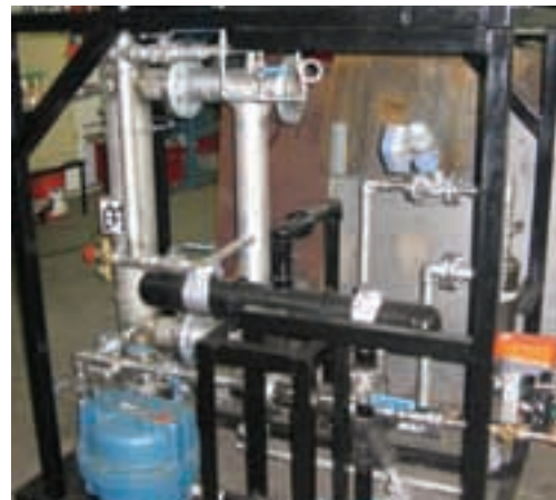
Humidification / sterilisation Steam to steam: 1400 lbs/hr Steam supply @ 110 psig ; Back pressure 15 psig Floor space 9' x 4'
